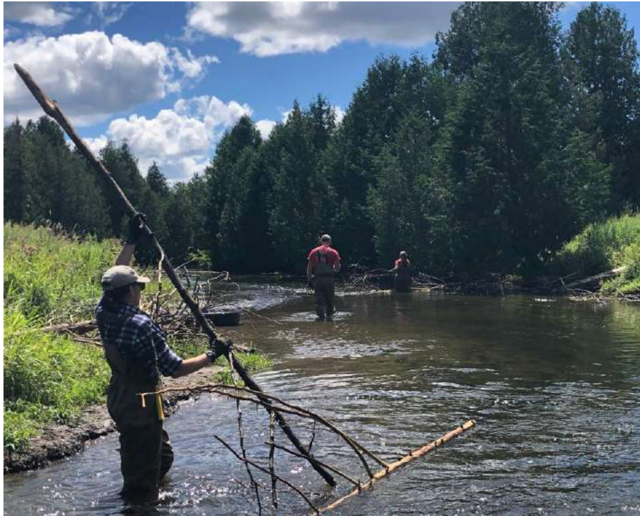
August 10 - Bringing large cedar logs downstream to be positioned in place (before installation)
